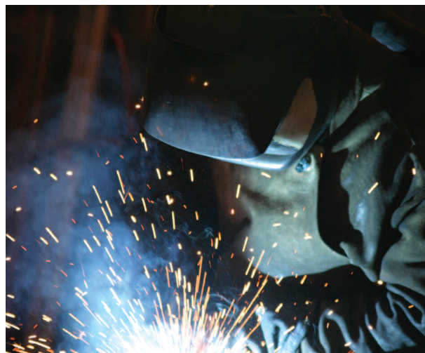
A welder at work at Newport's Rowecord Group, one of the eleven Welsh-based companies featured in Roaring Dragons . The Group, which employs 1,000 people, designs and creates complex steel structures such as the iconic 140 metre long cable-stayed foot and cycle bridge that has become the centrepiece of the SA1 development in Swansea.
